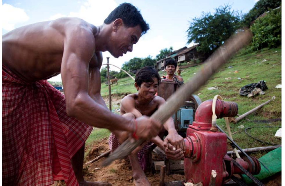
Villagers are setting up a water pump machine / Photo: The Asia Foundation
