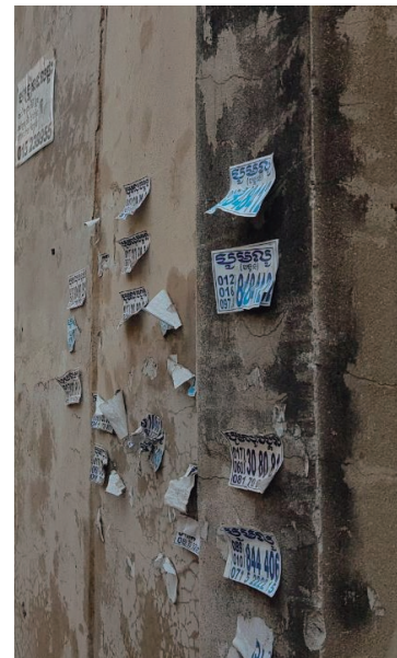
Figure 58: Plumber Posters on the wall.
